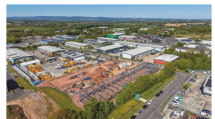
▲ The construction of the steel frame for eight of 16 planned industrial units at Westpark 26 Business Park in Wellington.
